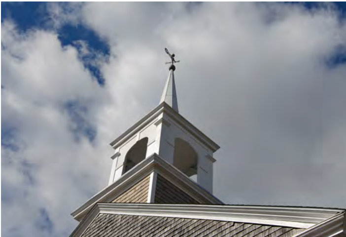
The East End Meeting House's steeple, which was added in the 1840s, was replaced with a fiberglass replica in the 1980s to alleviate pressure on the roof.
