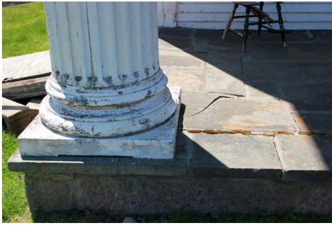
Detail of column base and porch. A crack can be seen on the porch.
