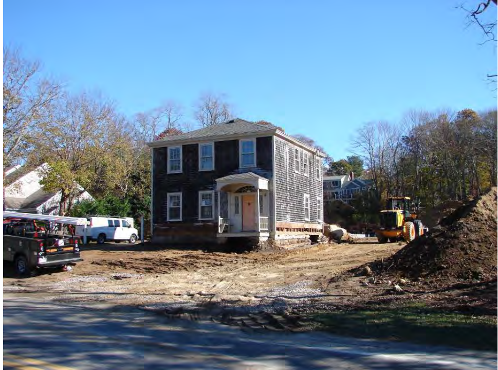
Recent condominium project under construction. The historic property was destroyed, including a nineteenth century barn. The house was stripped and inappropriately treated. The project had a significant adverse effect on the integrity of the historic district and the village.
